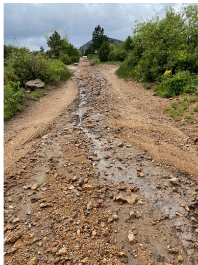
Road damage due to heavy rain
